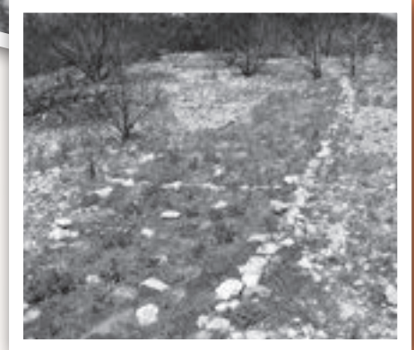
Straw erosion and seed mats were laid. After six months, results are evident.
